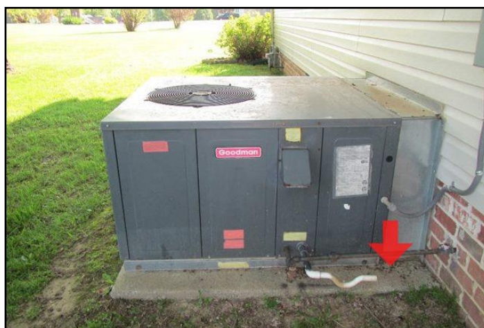
Improper discharge point
