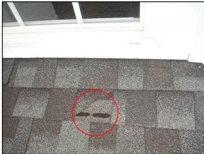
Missing, loose or torn
