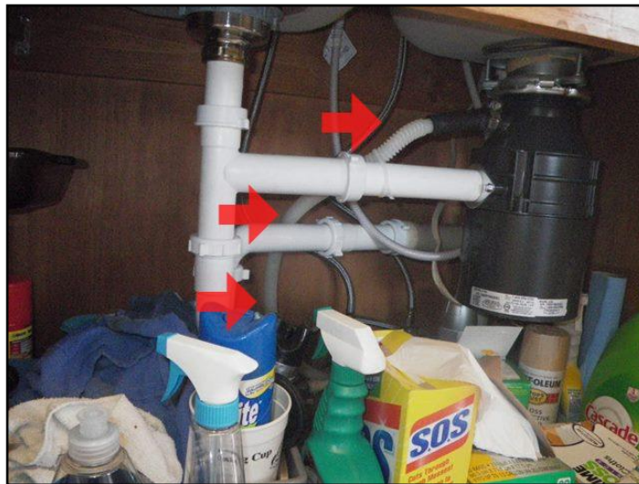
Backflow prevention missing
