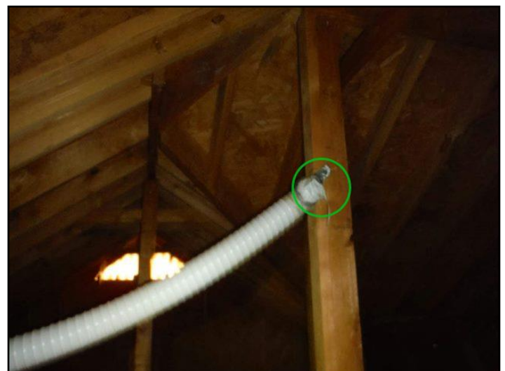
Poor termination location
