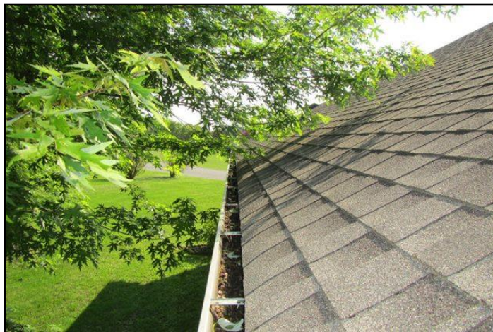
Trees or shrubs too close to building
